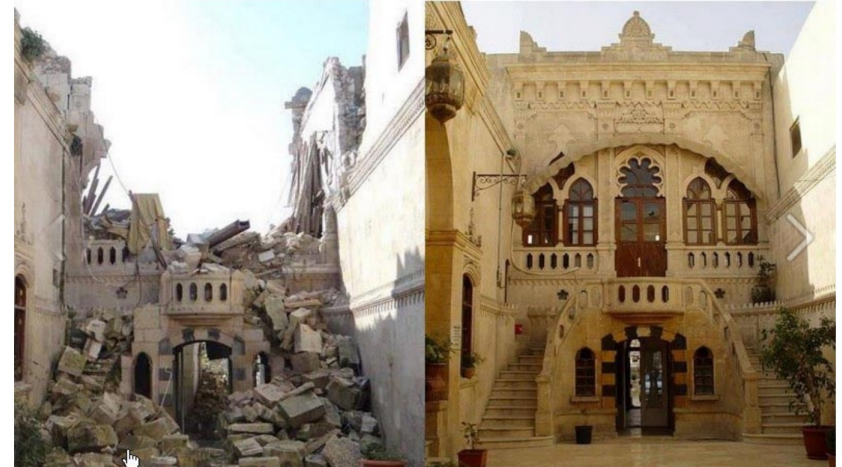
Figure 20: Example of damage to an intricate building - the fallen stones are visibly recognizable
