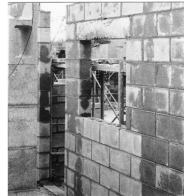
(b) Water from the Fluid Grout is Absorbed into the Block and Results in Surface Wetness (Courtesy of Gary T. Suter)
