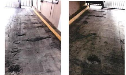
Figure J2: Spalling with exposed steel reinforcement at topside of garage deck.
