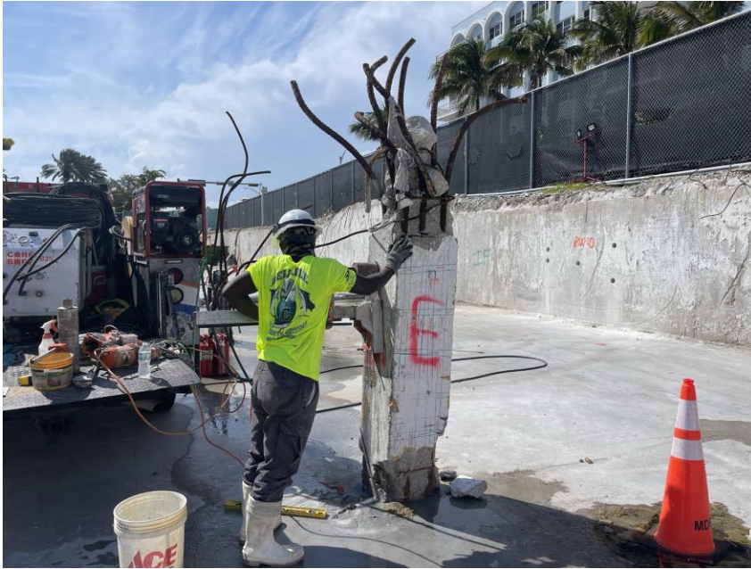
Concrete core collected from a column
