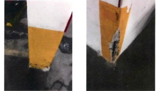
Figure J1: Typical cracking and spalling at parking garage columns
