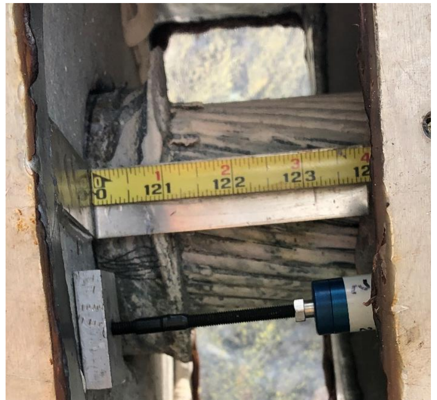
A4N AUX showing 7/8-inch extension (September 2020)
