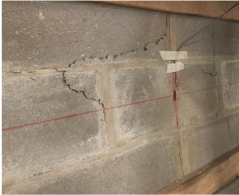
Masonry Crushing Compression-Controlled Section
